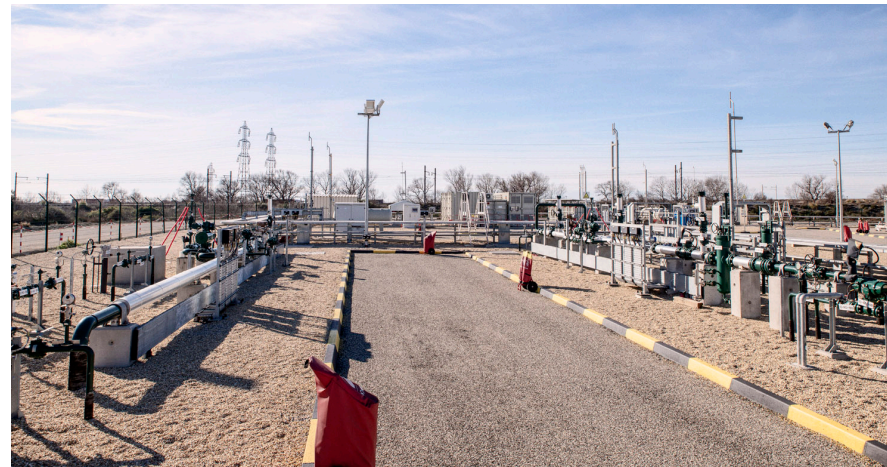
Hydrogen is injected in the grid since 02 2020
