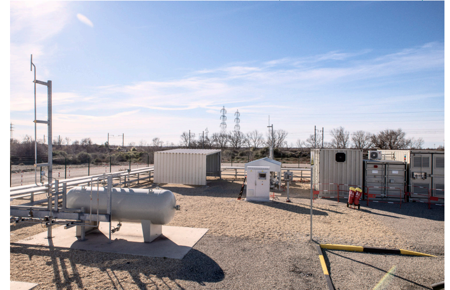
The methanation device is settled
